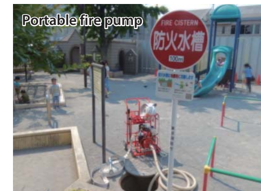
This motor-driven pump sprays water drawn up from a "fire prevention water tank" or similar water source.
