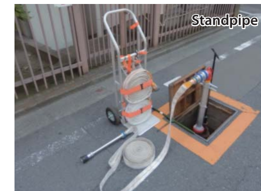
Connects to a roadside fire hydrant and utilizes the pressure to spray water.
