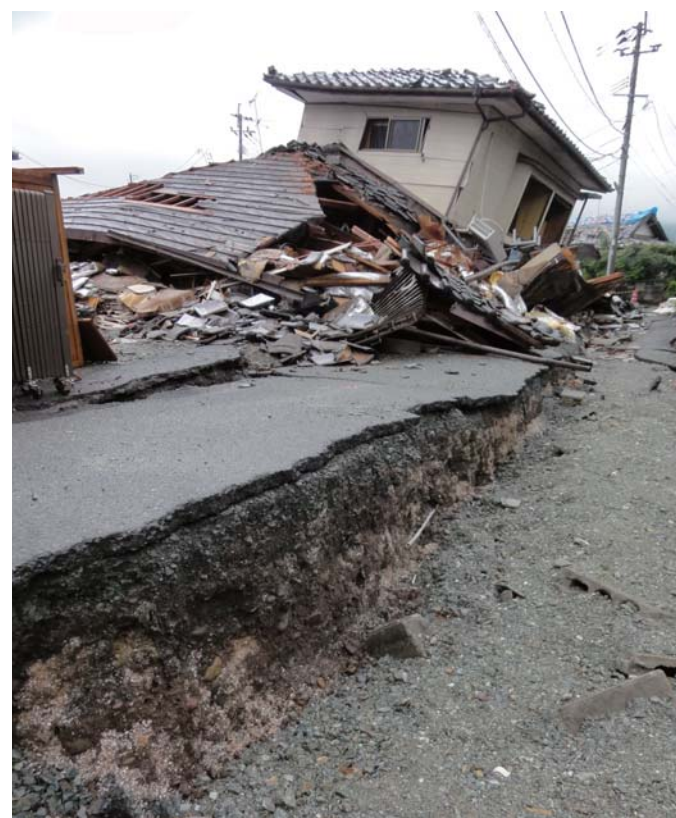
A collapsed wooden house atop a massively cracked road (Town of Mashiki, Kumamoto)
